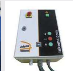
The control panel is installed beside the door
